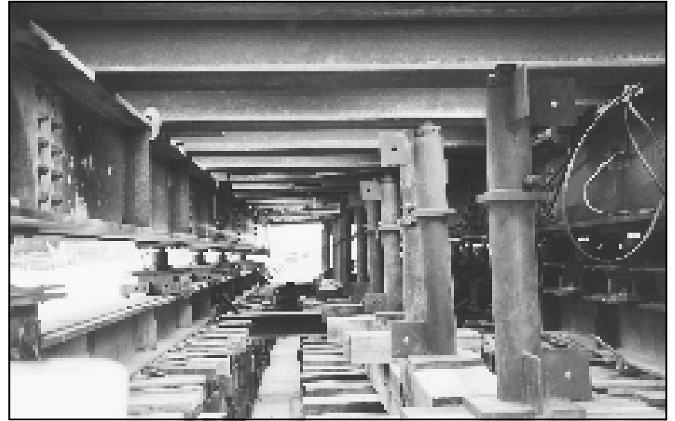
▲ Figure 26. Steel shoring towers in location for removal of rollers/travel beam and jacks.
