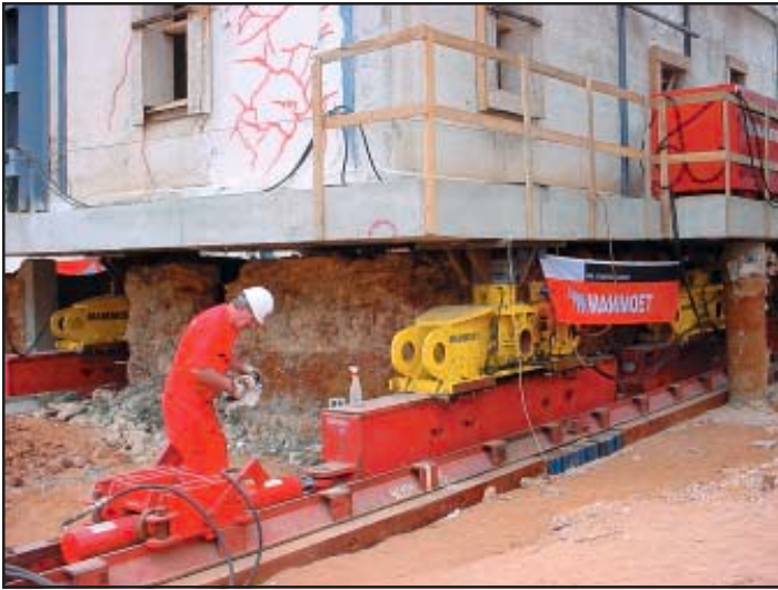
Mammoet used their computer controlled hydraulic jack-and-skid shoe-and-beam assemblies with hydraulic push/pull propulsion and standard track to move the structures.
