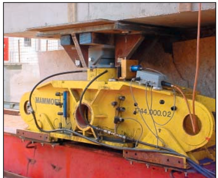
A detailed look at Mammoet's jack-and-skid shoe-and-beam assembly reveals the electronic control and measurement systems installed feeding the central computer.
