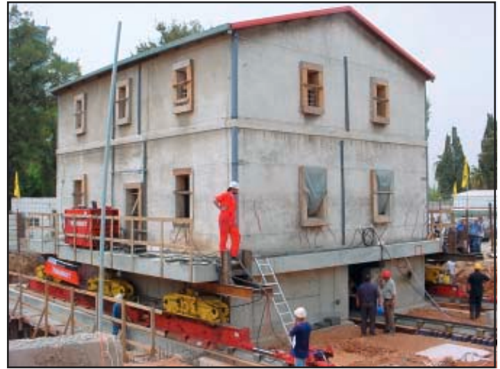
A structure was skidded to and over its newly built concrete cellar and lowered by means of the inbuilt jacks in the jack-and-skid shoe.
