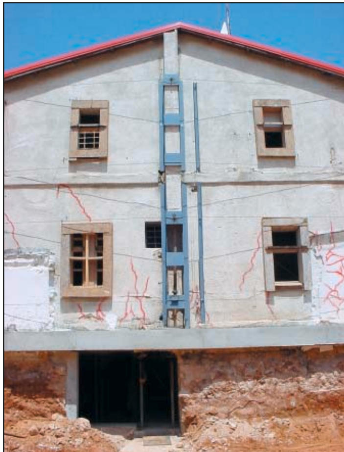
The fragile Templar houses required additional strengthening and shoring up, together with an additional concrete floor, to enable jacking and skidding.
