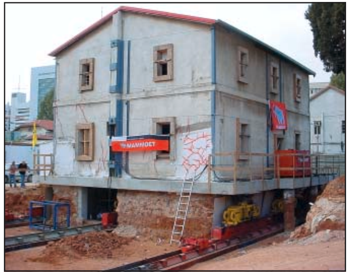
The Templar houses were excavated around in order to clear the cellar and to enable the Mammoet crew to install their skidding tracks and jack-and-skid shoe-and-beam assemblies.
