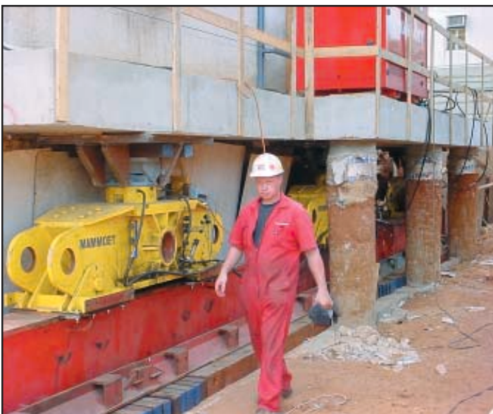
This Templar house had only a partial cellar underneath requiring additional piles to support that part of the additional floor in order to clear the ground underneath and to install the skidding equipment.
