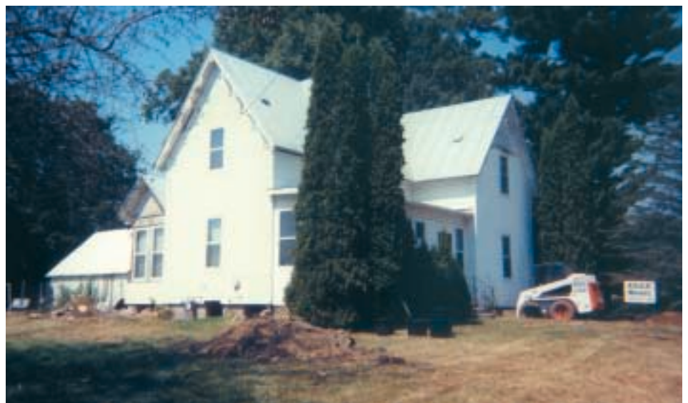
This 60' x 60' structure in West Salem, WI was elevated for a new basement, that was dug by the excavating company.
