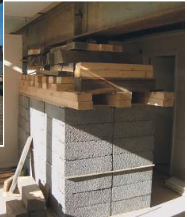
One of the four cribs with the beam resting on rollers closest to the camera and a Wetter air jack in place on the far end of the crib.
