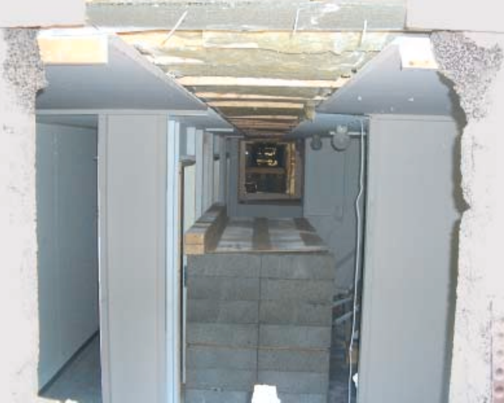
One of the two holes with one of the four cribs on the floor in the basement. We had also removed the boards from the ceiling to reveal the floor beams.
