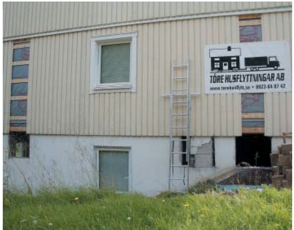
Holes for the two main beams are finished, including on half-made hole that was cut in the wrong place due to a drain freezing.
