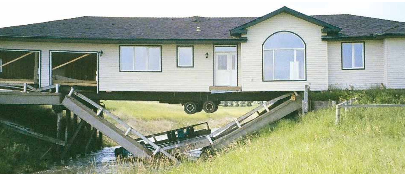
The dollies under the main part of the house were still on the bridge when it fell. The 90-foot beams saved the structure from going into the canal.
