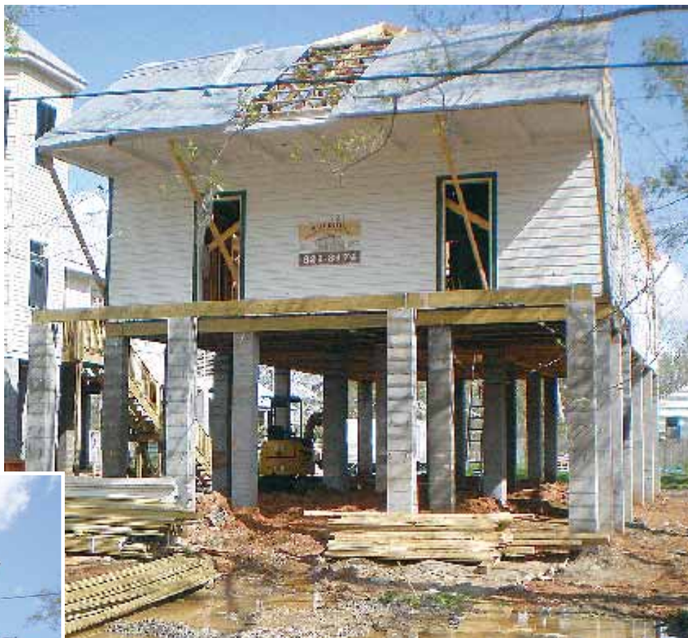
This 24 foot x 32 foot was pushed four feet off its foundation.
