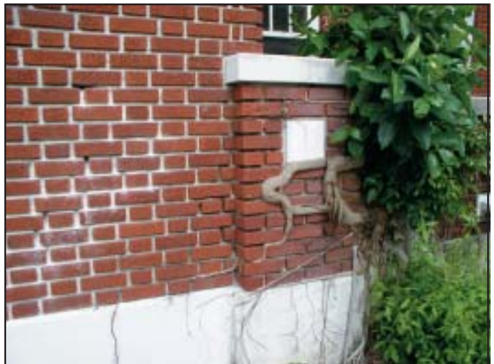
Non-use and no maintenance for eight years left foliage to find its own way. Cracks in walls were evident in several locations.
