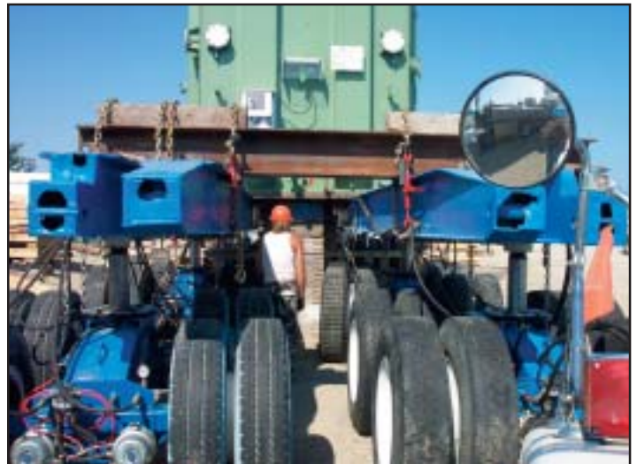
Due to unusual physical constraints equipment had to be modified while performing movement of the transformer.
