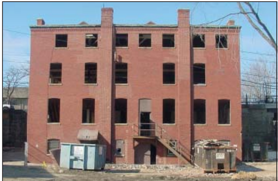
The building prior to beginning of construction. Note stairs leading to the first floor. The ground level is used as a basement.
