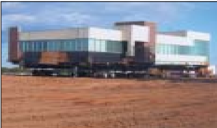
Power dollies were used to move the building approximately 3/4-mile across a field and highway to a new site.
