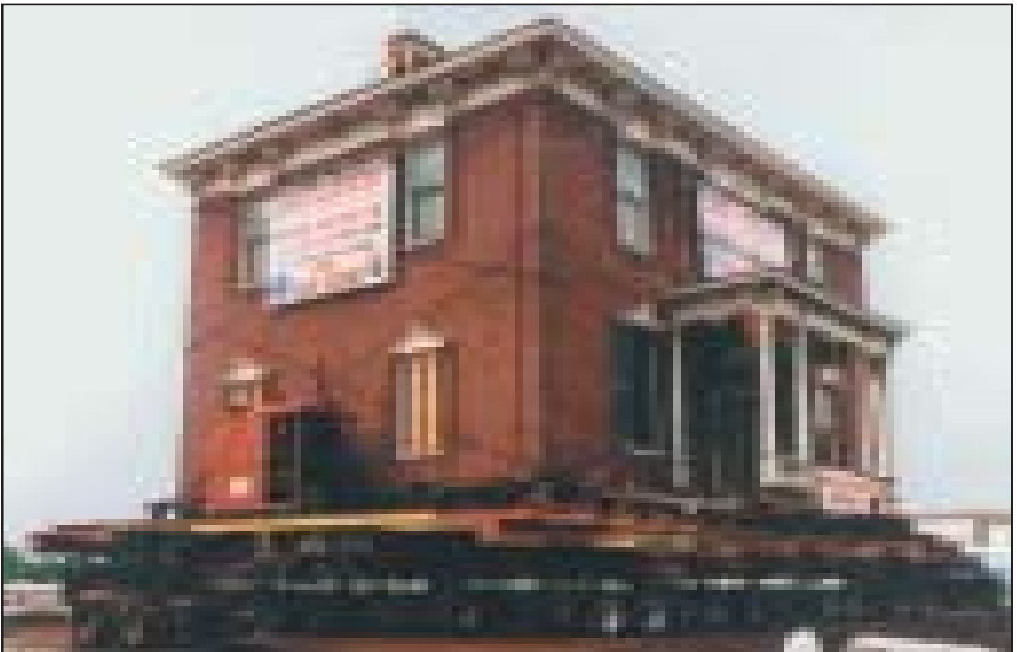
The 175 years old structure is 60' L x 48' W x 52' H, weighs 562 tons and is listed on the National Register of Historic Places.
