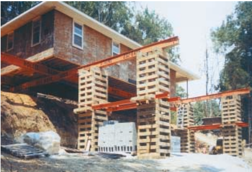
Relocating a residence to a mountainside plot required 18 feet of cribbing for slide beams to build a basement.
