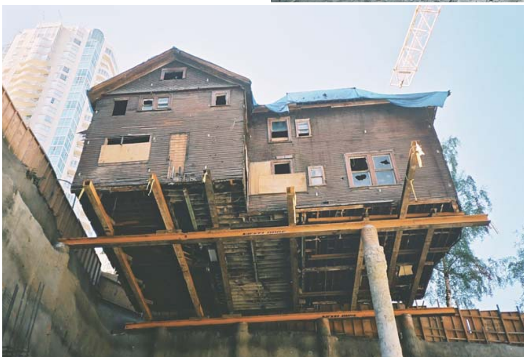
Building situated at the corner of the project with cross and main beams in full view.
