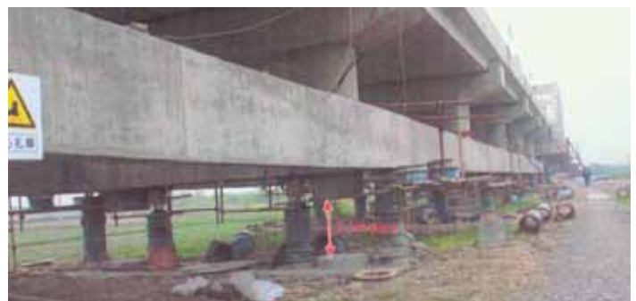
Hu-Ju-Shen Land bridge, and weighing 3600 tons, during raising (May 2004) Lianshi, Huzhou. Raised 2.5 metres. Note the form of cribbing used (May 2006)
