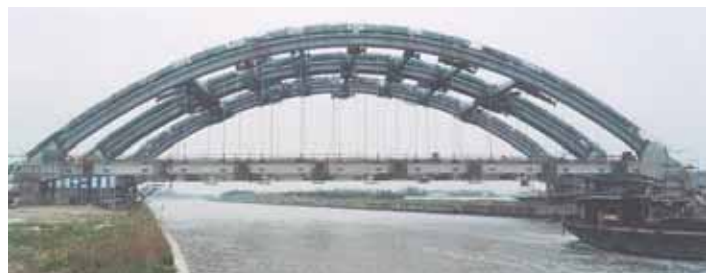
Wusong bridge with a span of 85 metres and weighing 3600 tons, during raising (May 2004)
