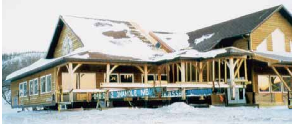
A view of the overhanging roof. Beams are supporting a veranda. The first of three cuts dividing the building is clearly visible.
