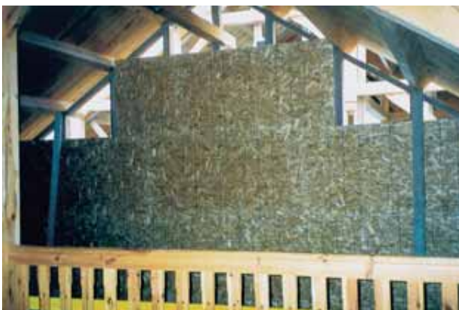
A view from the loft area of the temporary wall built to support the weight of the roof.
