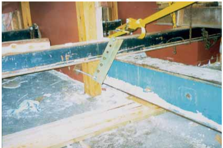
Wooden posts secured to crossbeams and main beams with angle iron. This, also, was used to minimize cosmetic damage and maximize overall structural stability.
