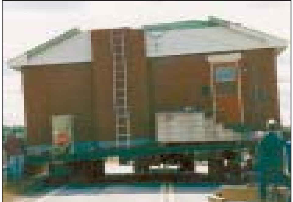
A method to cut the bonnet (cap) of a structure allowing minimal reconnection time saves thousands of dollars in utility crews costs. The process allows for slicing each truss, or rafter, and replaces two rows of shingles. This increases the speed of the move 10 fold and often permits delivery of the structure set in place in one day. The roof, is transported on an air-ride float behind the house during the move, and can be set in less than two hours on a standard house using a small contractor for reattachment. Bracing leaves the roof stronger in some structures.
