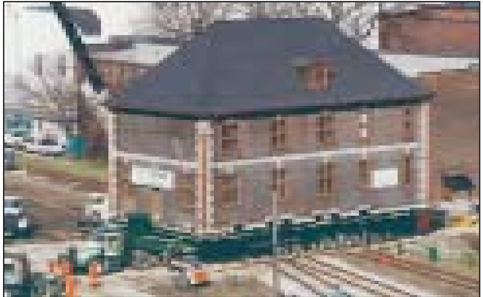
In 1944 we moved this building that was constructed in 1904 over the foundation of a church that was the original town hall of Walkersville, now known as Windsor. The structure, on the property of Hiram-Walker Distillery, was moved for the Walkersville Historical Society as a heritage (historical) building and became an art gallery at the new location. Total tonnage, with steel, was 750 tons, 158 tons on the fifth wheel of the 1980 Auto Car tractor with a 65,000 planetary rear-axle. The truck was originally used to move 100-ton steel ingots at the Defasco Steel Mill in Hamilton Ontario.
