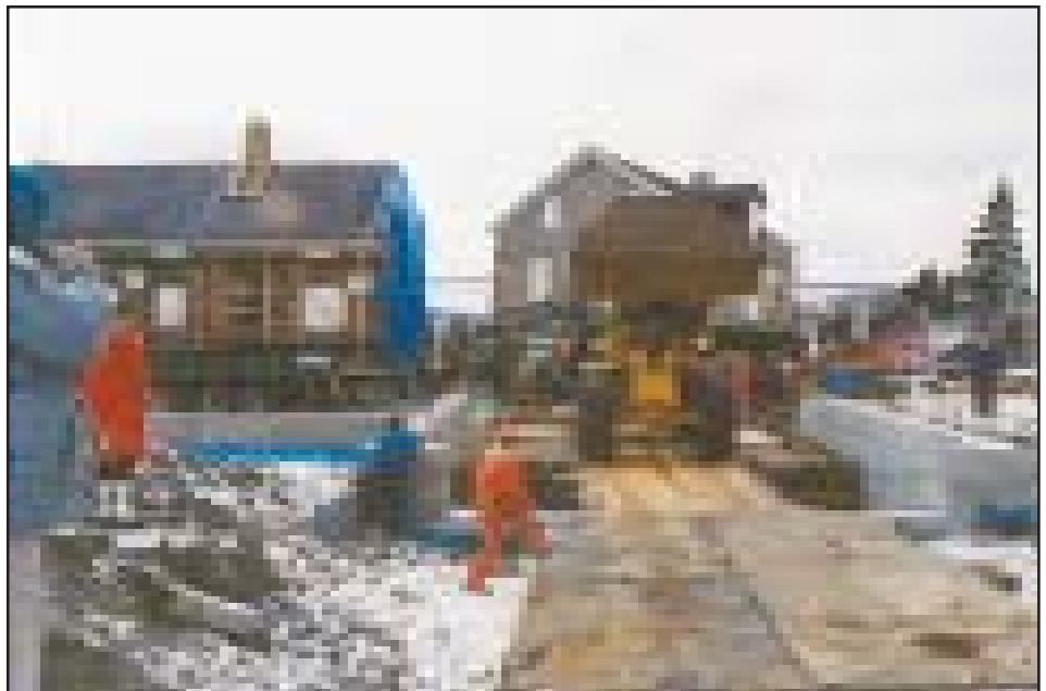
Woodhouse Museum in Cornwall on move day. A hydraulic lifting bolster beam permits side shuttle and lifting over and setting down on the new foundation.
