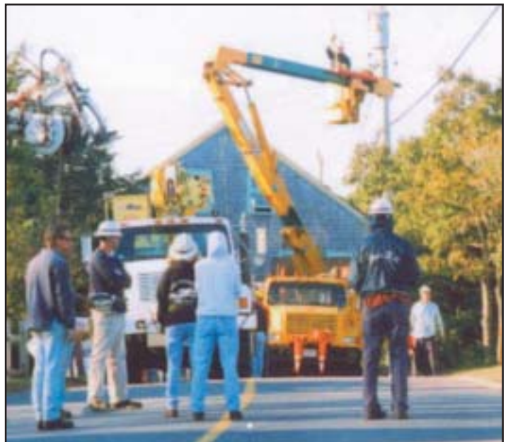
Elevating utility wires and removal of roadside obstructions are common elements that must be overcome when moving most any large structure.
