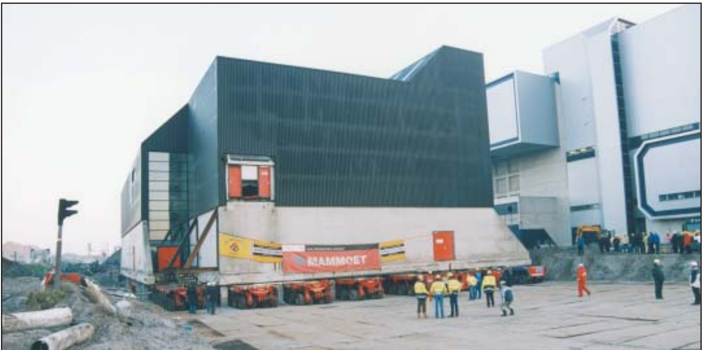
Early Saturday morning the building was lifted free from the remaining foundation piles. Keeping all wheels on the plates and keeping the SPMTs from not interfering with the remaining piles required keeping a close eye on all trailers.
