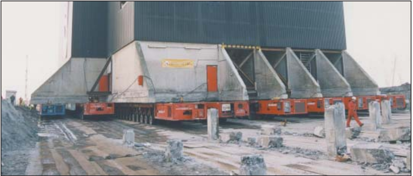
Despite drainage and weight spreading steel plates the enormous impact of the weight became clearly visible as the ground water came up.
