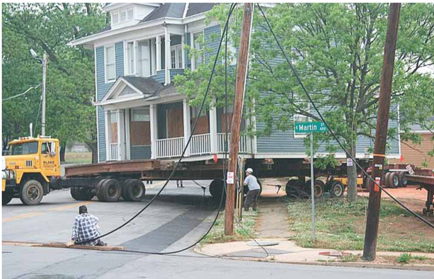
Blake Moving Company simultaneously relocated eight houses in downtown Raleigh, North Carolina in 2007.
