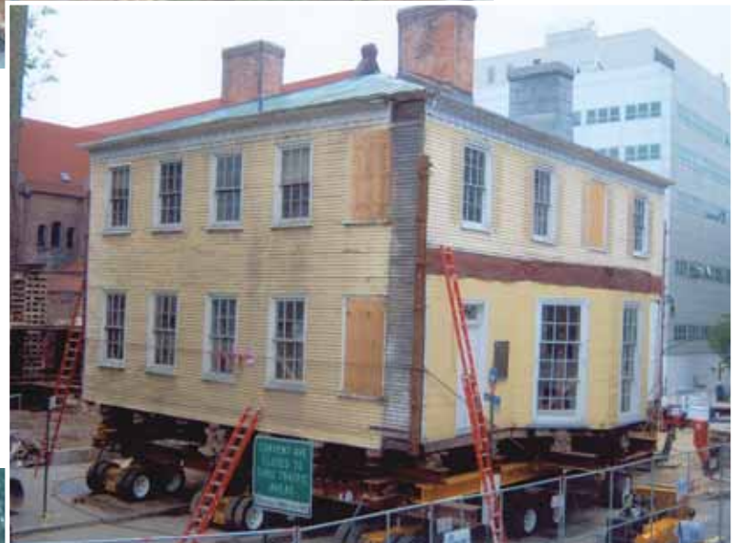
Installing the bracing in preparation for the trip down the street and the 9° grade.
