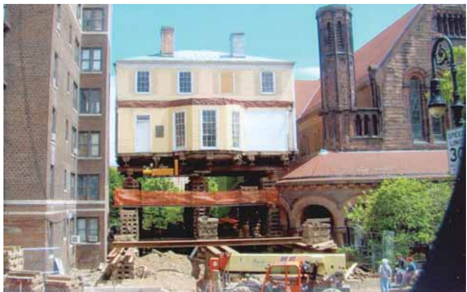
Getting close to the 40-foot above ground level necessary to clear the portico. The street was about five feet above the ground level at the house.
