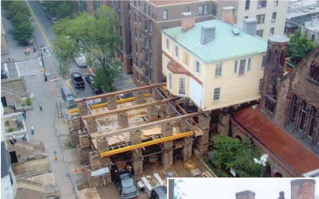
Sliding the Grange out across the portico. The building is 35 feet above street level in this photo.
