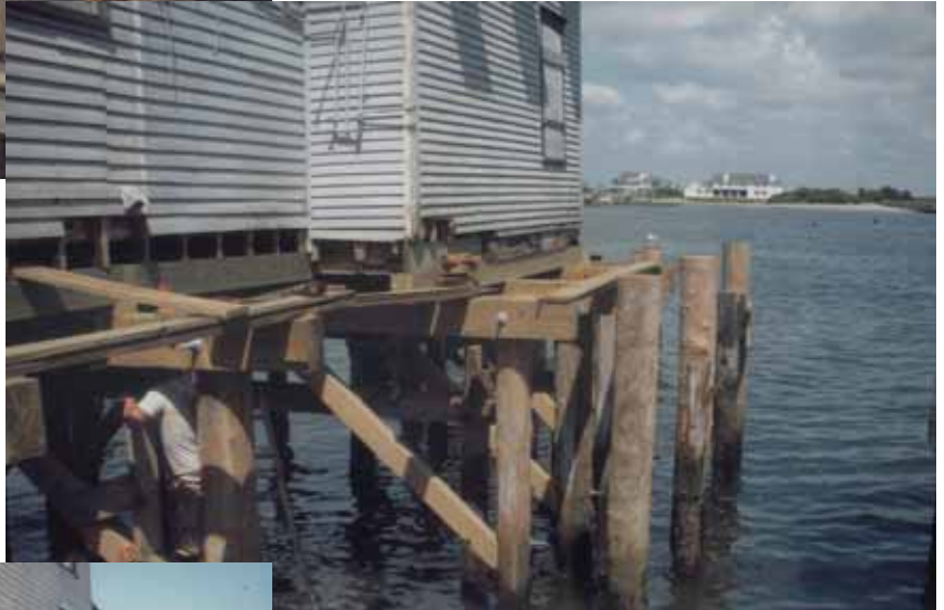
Stringers bolted to new pilings and excess cut off. (Crew Installing Supports)
