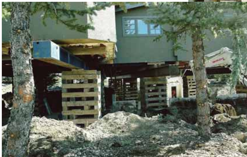
A view of the piers from the outside and shows where one of the additions joins the main structure.
