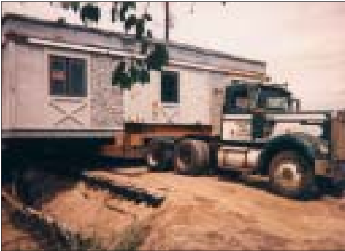
This restaurant was elevated seven feet while situated on five feet of sand and 34' of muck in South Carolina near the Georgia border at Savannah. The road had to be reinforced for passage.
