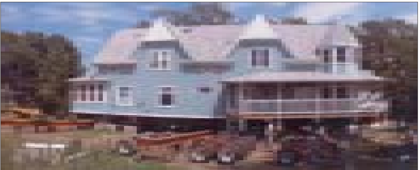
Three rolling beams carried the structure onto six Telkamp AutoSteer hydraulic dollies to transport the load.
