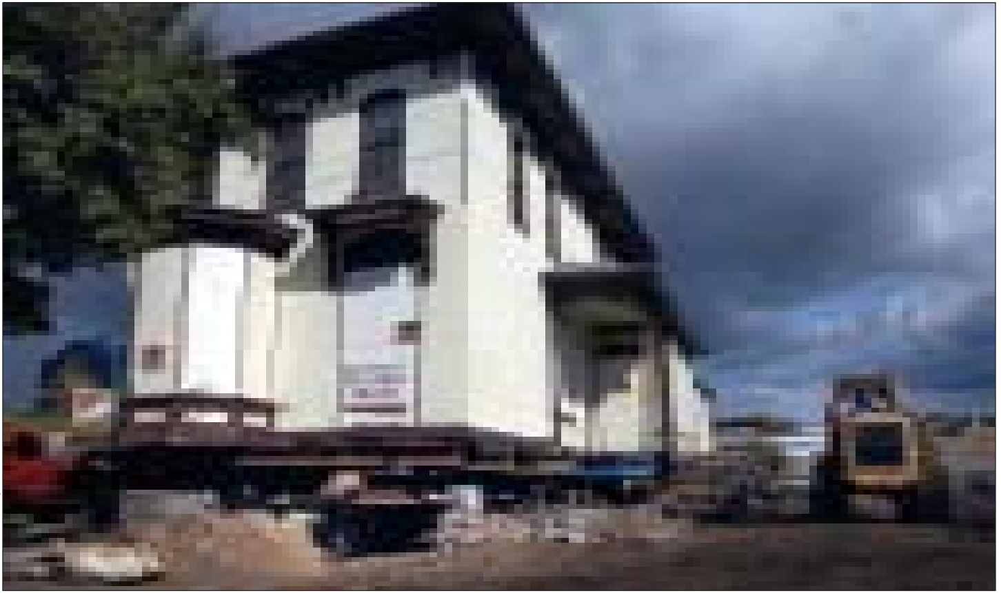
Upon Blocks: The former home of Tom Kroon has been lifted from its foundation in preparation for the move.
