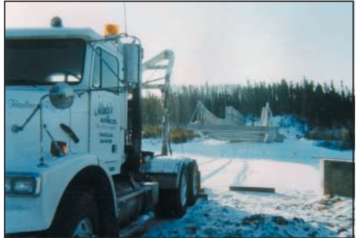
Our winch truck on north side of north abutment. (Note nose section pointing up to counter act launching droop.)
