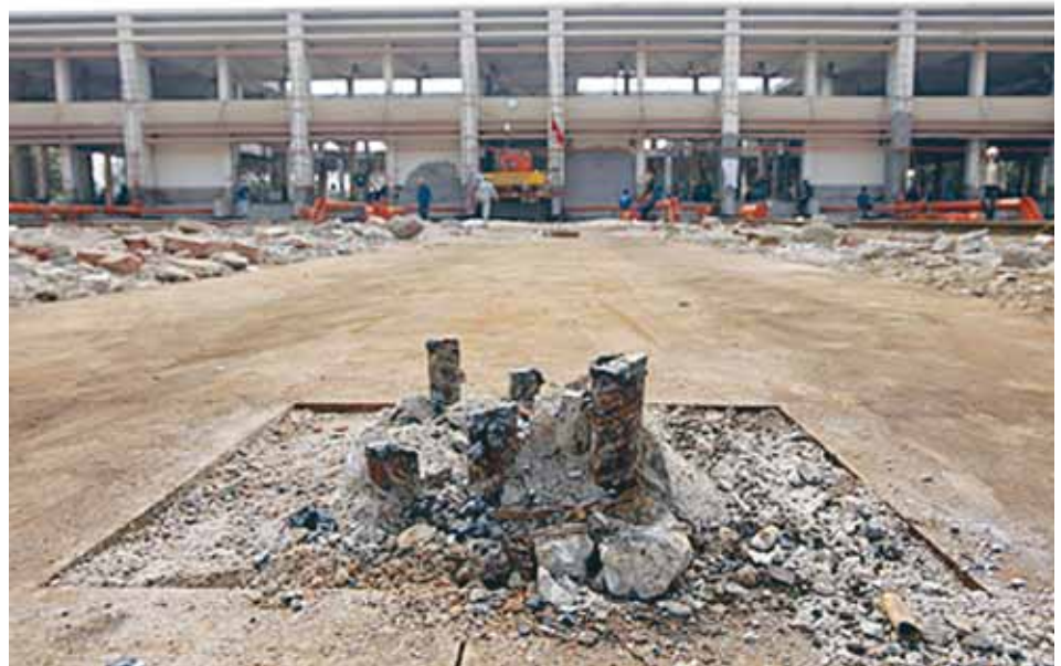
This photo is of the front of the building. Notice the "pushing cylinders in orange. This was the last day of the "pushing" process. The object in the foreground is the remains of a pillar of the original foundation. The pillars were cut and the building was placed on rollers. The building contained 88 pillars
