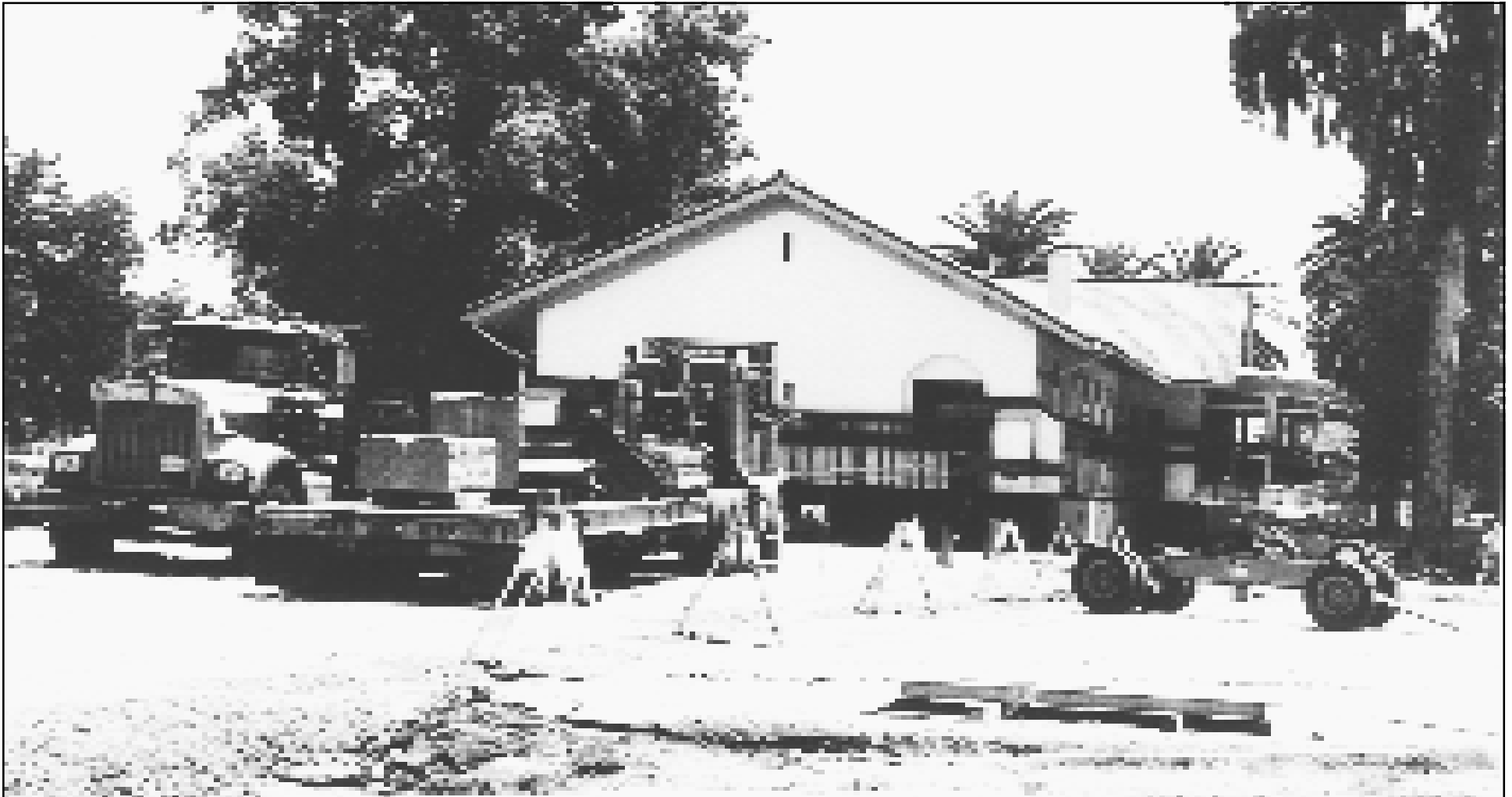
As the hospital wing is being pulled off the former foundation, the crawler dollies are being exchanged for the rubber tired dollies.
